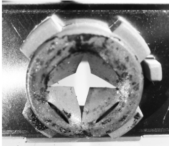
It is necessary to replace
